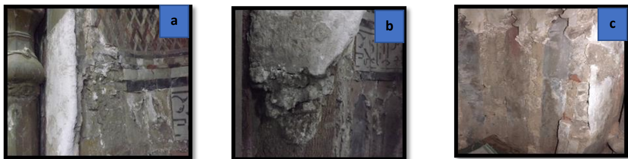
Fig. (4), falling off layers of stone cladding, a, Falling layers of cladding from the left side of the mihrab, b, Close up of the previous photo (a), c, Falling layers of cladding from the bottom of the mihrab
