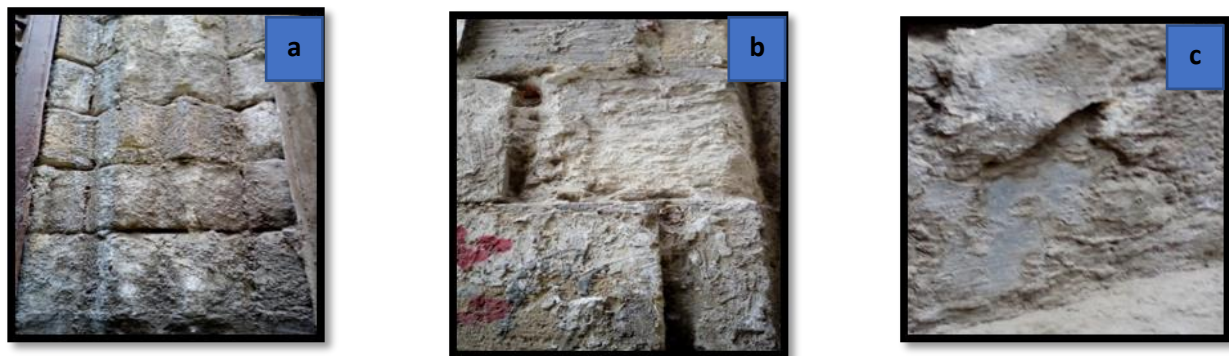
Fig. (3), Weakness of the bonds between the mortar and the stone,a, Describes the fall of mortar layers, b, showing the worn out parts of limestone,c, buckling layers of limestone
